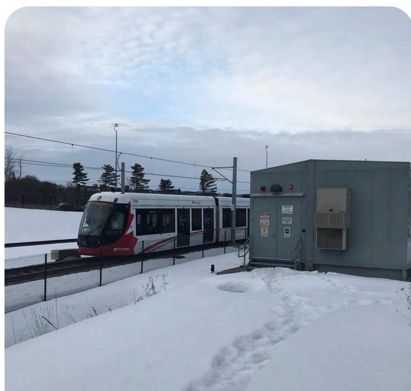
Power Substation Ottawa LRT
